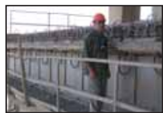
Application, TORK Pulse Valves
